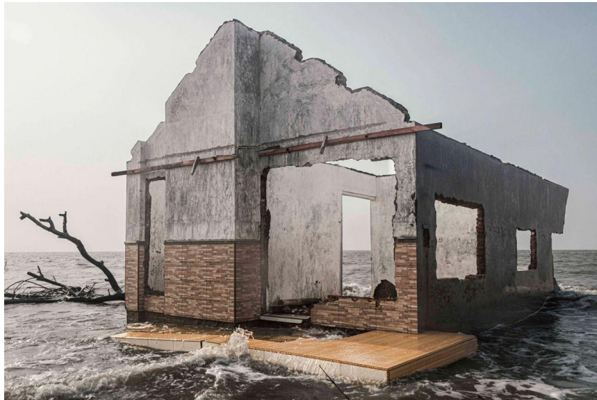
Image 1. A deserted house stands out in Java Sea Pekalongan; coastal floods have submerged the settlement. Indonesia. Barlian, Irene. 2021.
