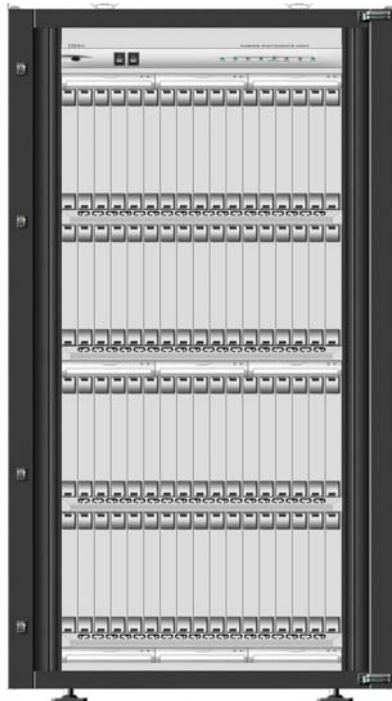
Gambar 2 Rack Mobile Switching Center
