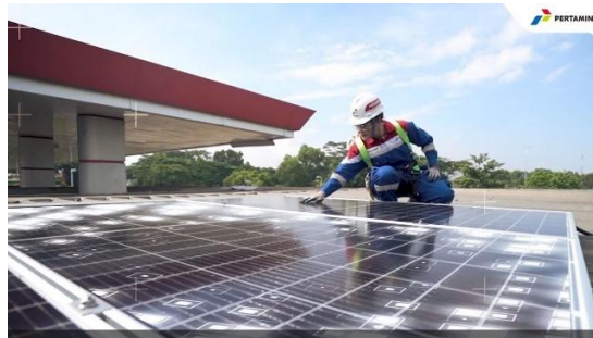
Figure 3 Solar PV in Pertamina's Gasoline Station
