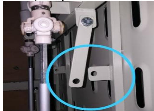
Figure 5. There is a Coating Defect
