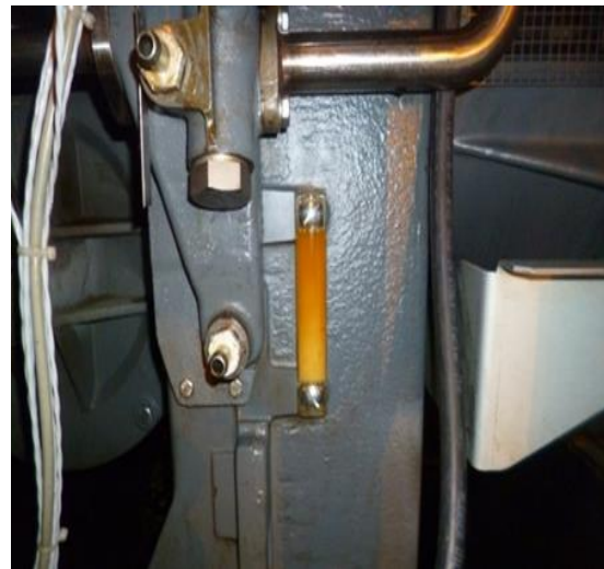
Fig. 2. Visual examination of the oil in the screw compressor
