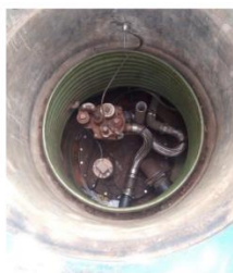
Fig 1. Pertamina storage tank
