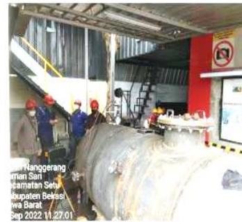
Fig. 1. Air receiver tank.
