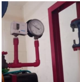
Fig. 3. Pressure Indicator on Pressure gauge
