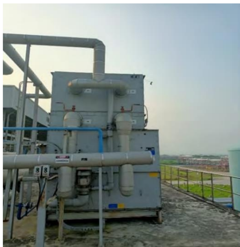
Figure 3. Condenser of the refrigeration system
