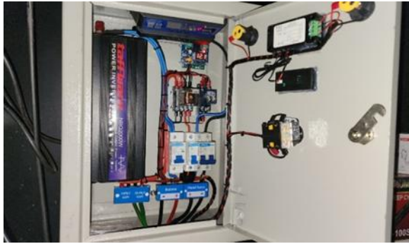
Figure 12. SCC control panel for solar panels
