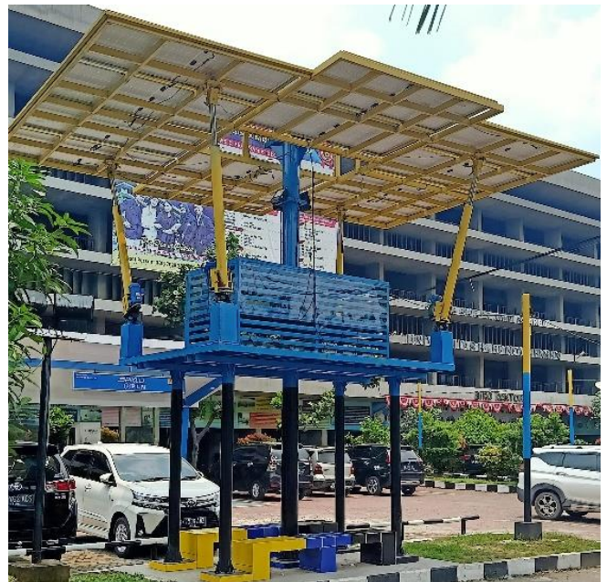
Gambar 1. PLTS Autotracking 5 KWP
