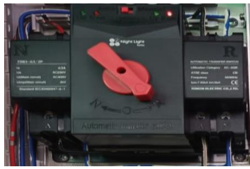
Gambar 4. Automatic Transfer Switch
