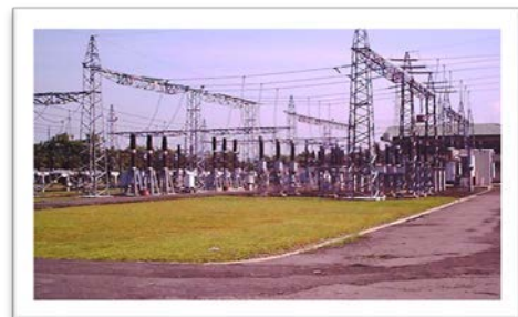
Gambar 1. Switchyard Gardu Induk Konvensional
