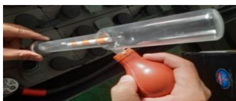
Figure 8. Battery Electrolyte Density Testing data collection
