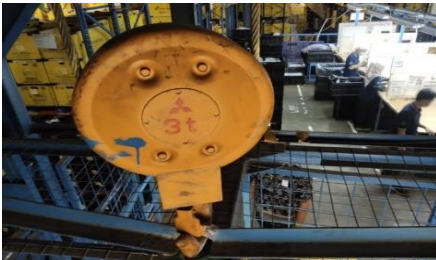
Figure 5. Goods Elevator Pully
