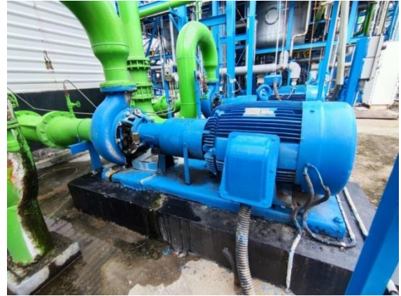
Gambar 4. Pompa sentrifugal cooling water P9114B
