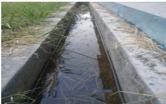
Figure 1. RPS TKRO SMKN 1 Ciruas wastewater channel
