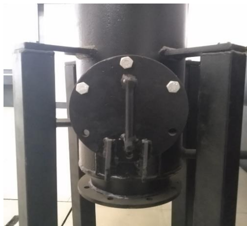
Figure 3. Hand Hole Valve Before Modification
