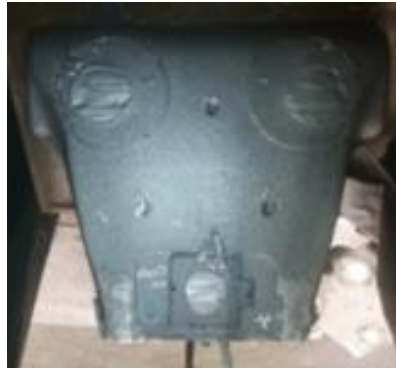
Figure 7. Surface of the bracket product after repair
