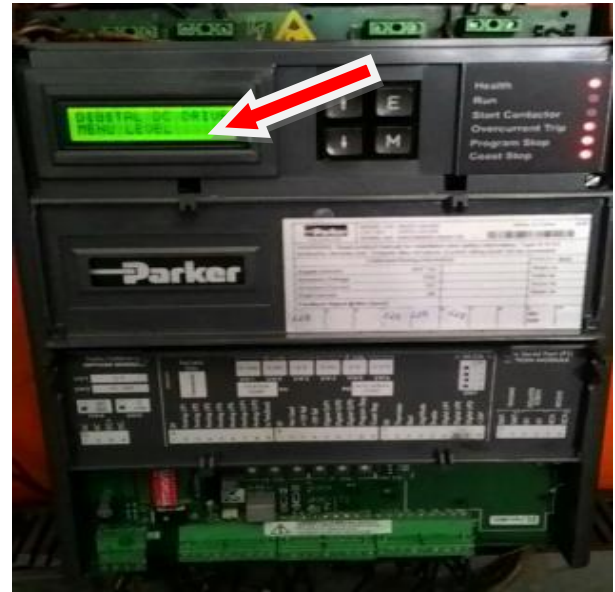
Figure 10 Digital drive control.
