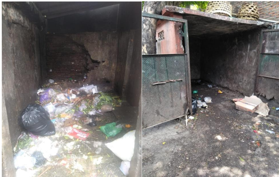
Figure 1. Garbage Bin at Sentul Market
