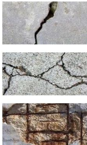
Figure 1. Examples of images with respected types of cracks, from top to bottom, early thermal contraction, plastic shrinkage, and corrosion reinforcement crack images
