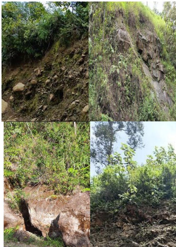
Figure 1. Slope surface condition
