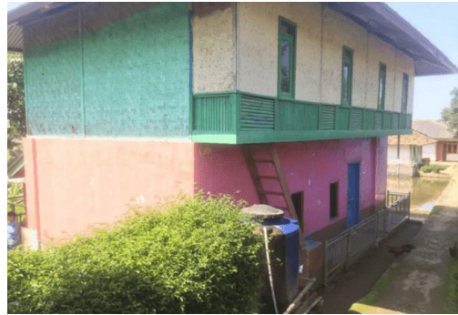
Figure 9. Side view of a two-story building that suffered moderate damage
