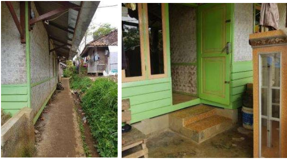
Figure 1. The house is earthquake safe because it uses a stilt structure and woven bamboo walls
