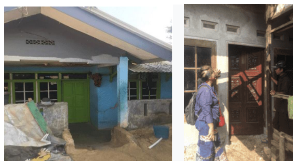
Figure 12. The brick house had damage to several sides of the building because blocks were not used in the building
