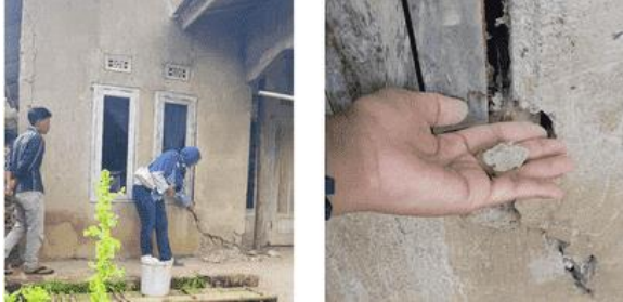
The house had brick walls without structural reinforcement so when an earthquake occurred, the house suffered damage and cracks on almost all of the walls of the building.
