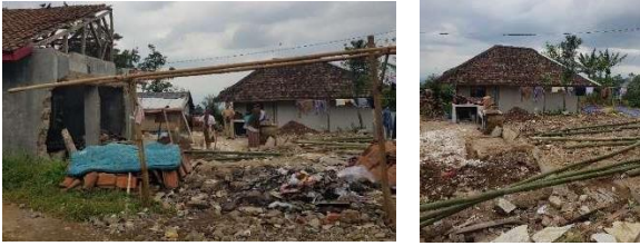
The permanent wall building in Cihikeu Village which completely collapsed
