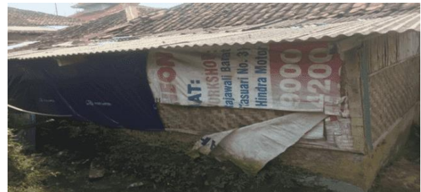
Figure 14. The addition of the building mass for toilet function can be seen behind the stilt house with woven bamboo walls
