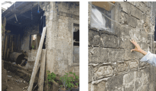
The house, which had brick walls without structural reinforcement, swayed when held Figure 10. The image above depicts a type II one-story house with brick walls without any structural reinforcement so that when an earthquake occurs the building suffers heavy damage.
