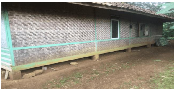
Figure 7. Side view of the Cihikeu stilt house building which uses a pile foundation umpak with materials dominated by wood and walls using woven bamboo
