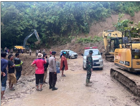
Figure 9. Landslide disaster in the road network area
