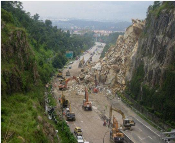
Figure 2. The rock slope failure incident at the Bukit Lanjan Interchange (KM 21.8 of NKVE) on November 26, 2003. The entire expressway was closed to the public due to the failure of materials obstructing the road [33].
