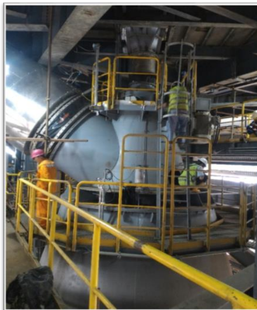
Figure 3. Photograph of Classifier – Coal Mill Measurement
