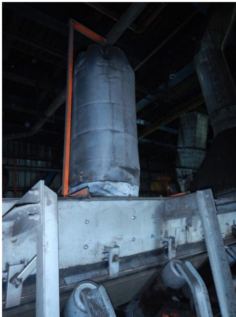
Figure 8. Dust bag at transfer point area of belt conveyor
